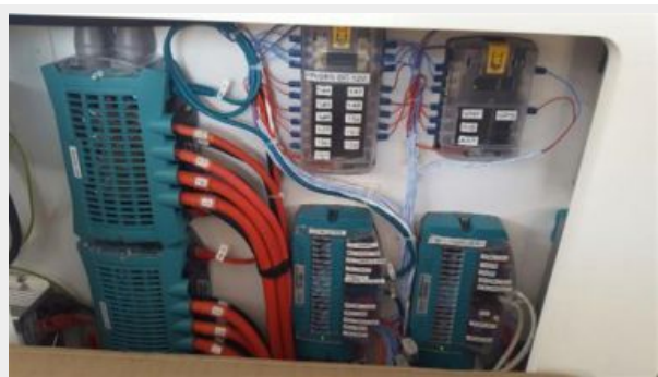
Electric System (Mastervolt)
