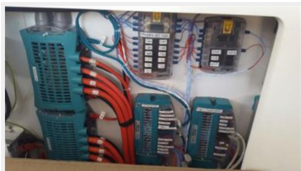
Electric System (Mastervolt)
