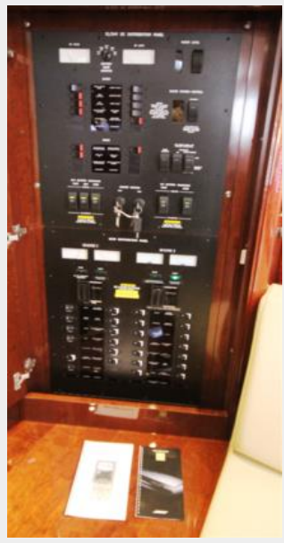
Main Distribution Panel
