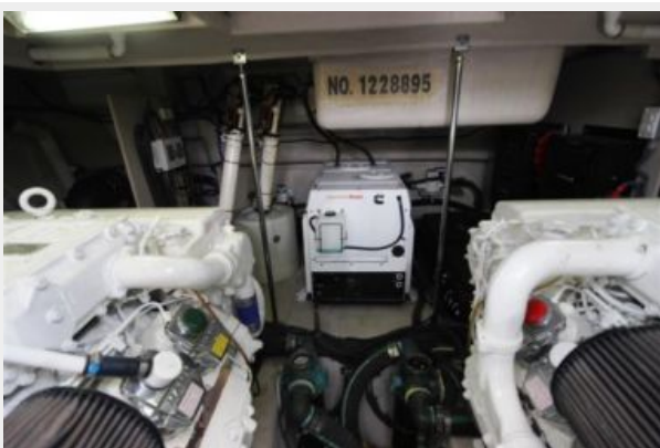
Enging Room Generator
