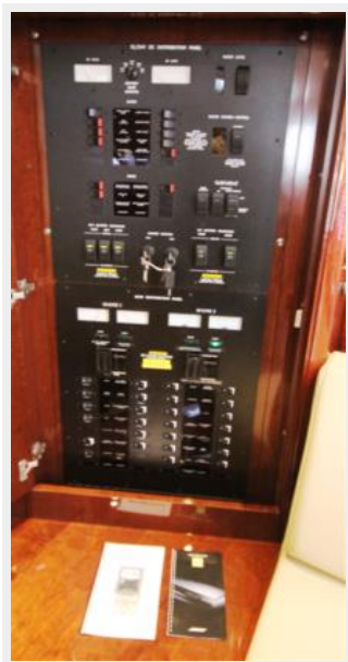
Main Distribution Panel
