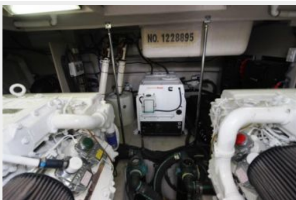
Enging Room Generator
