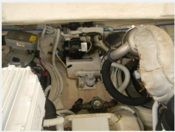
Engine Room Aft
