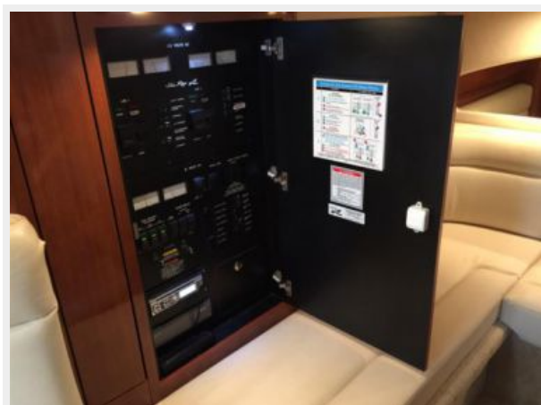
Main Distribution Panel
