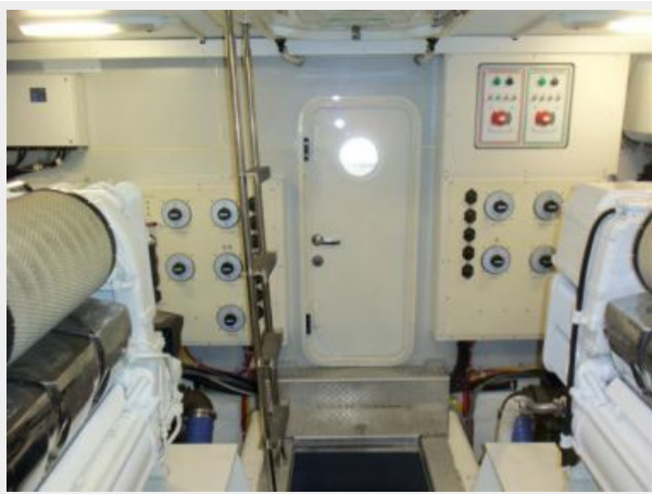
Engine Room Looking Aft
