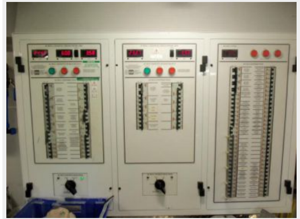
Main Engine Room Panel
