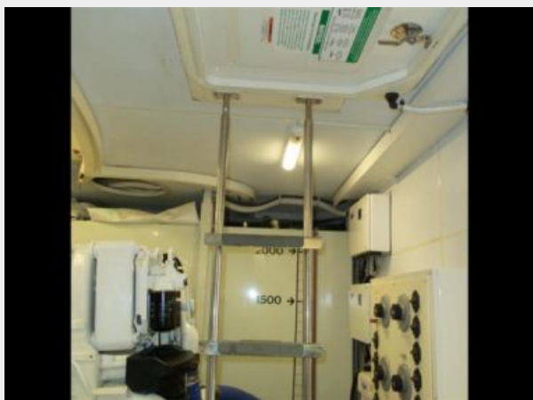
Emergency Engine Room Access
