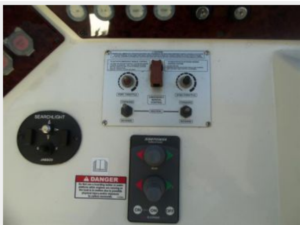
Backup Engine Controls & Thrusters
