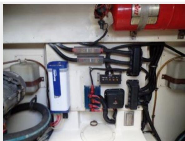
Engine Room Forward
