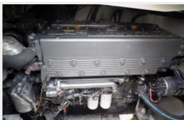
Engine Room-Port Main
