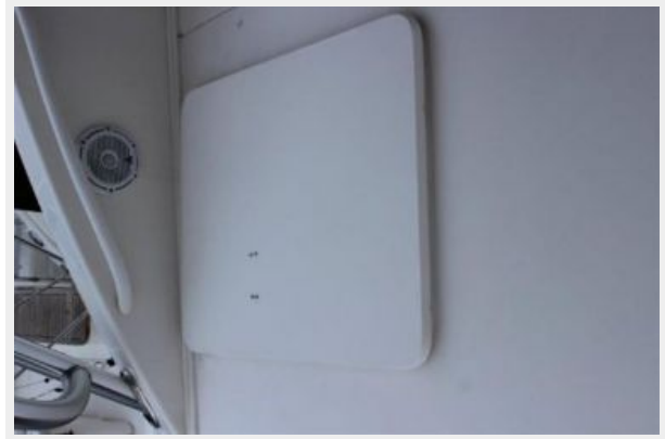
Deck 10 - Bridge Entry Cover
