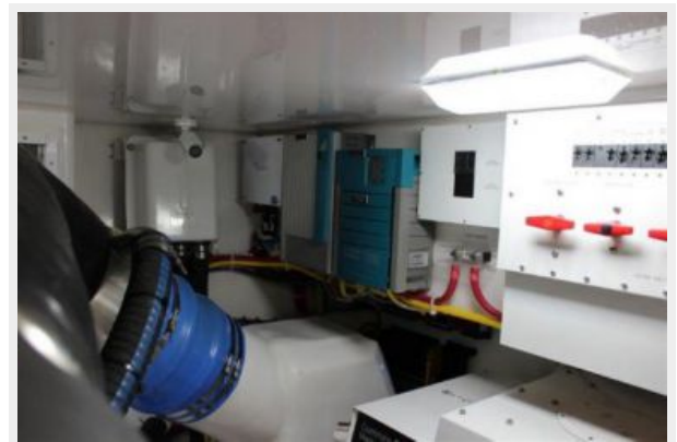
Engine & Mechanical Equipment 10 - Engine Room
