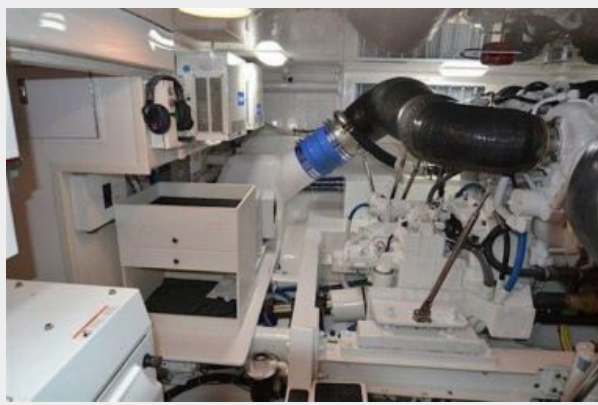
Engine & Mechanical Equipment 7 - Engine Room
