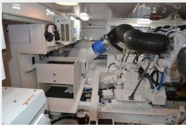
Engine & Mechanical Equipment 7 - Engine Room
