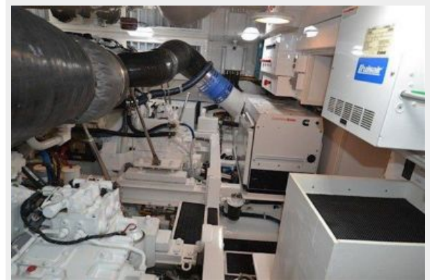
Engine & Mechanical Equipment 8 - Engine Room
