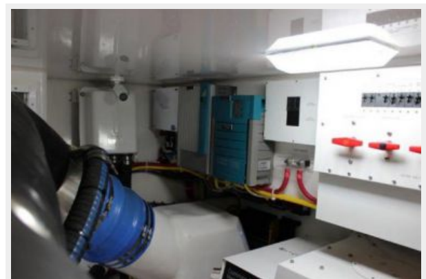
Engine & Mechanical Equipment 10 - Engine Room
