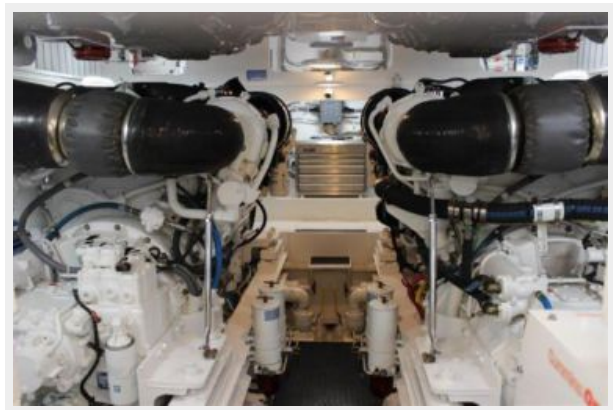
Engine & Mechanical Equipment 2 - Engine Room
