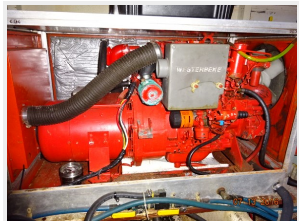
36' Grand Banks generator
