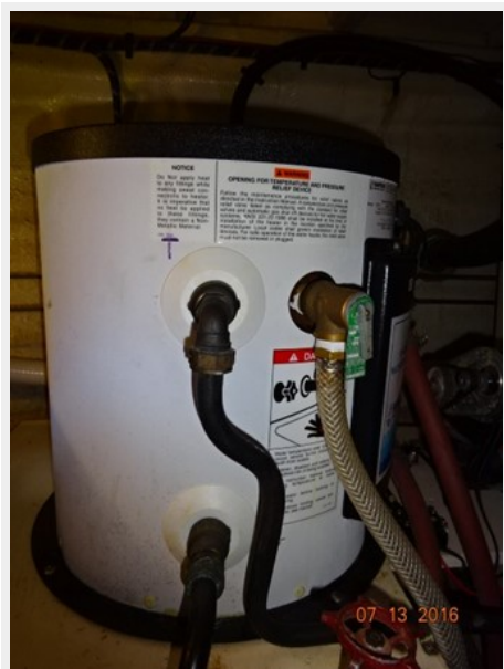
36' Grand Banks water heater
