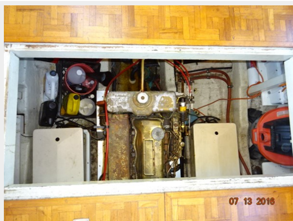
36' Grand Banks engine room access
