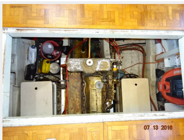
36' Grand Banks engine room access
