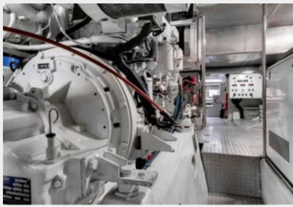
Engine Room (Note: Engine replaced with NEW John Deere, 2013)
