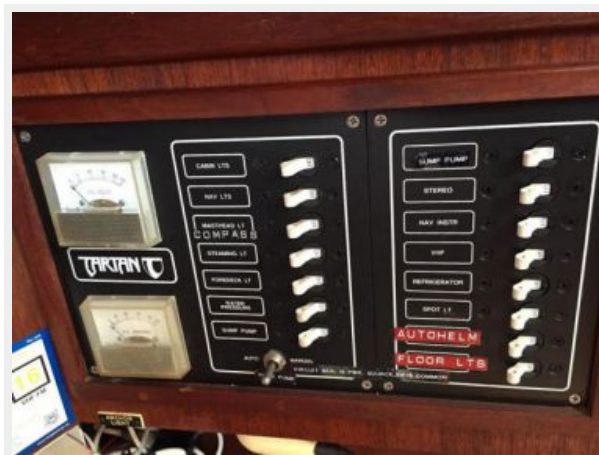
31' Tartan Electrical Panel
