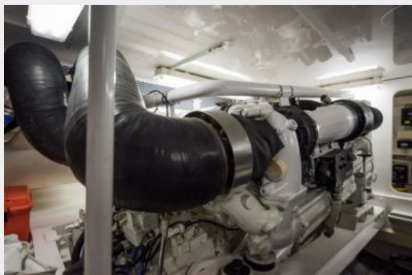
Viking 61' Enclosed Bridge - Engine Room
