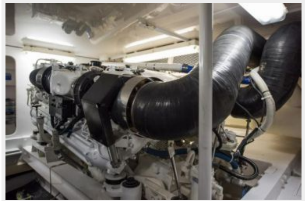
Viking 61' Enclosed Bridge - Engine Room
