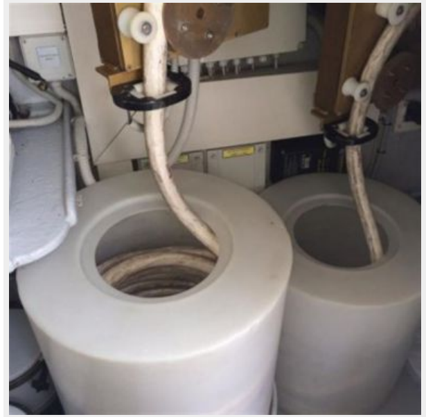
Cable master tubs utility room
