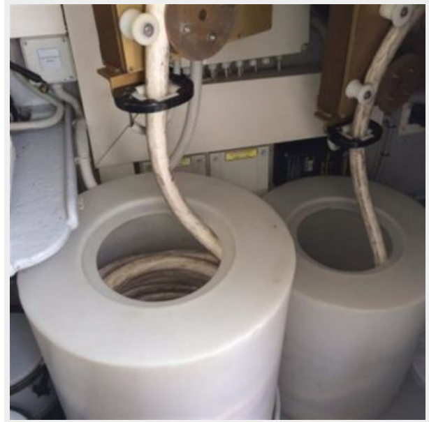
Cable master tubs utility room
