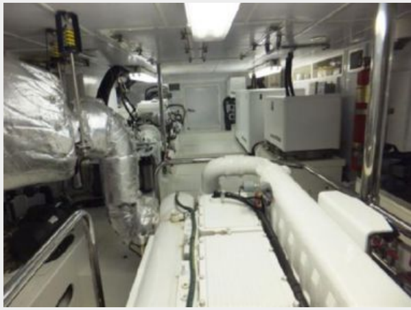
Engine room aft
