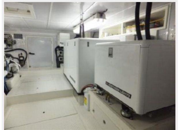
Engine room port
