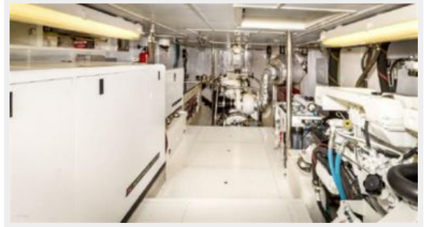
Engine room forward
