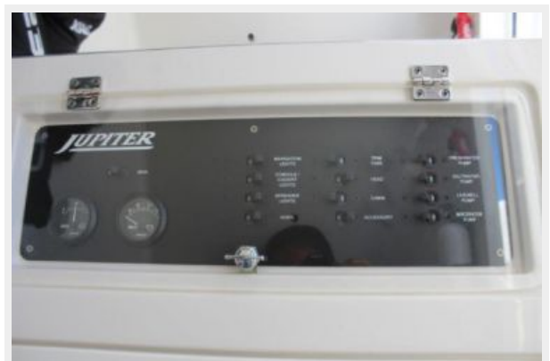
Electrical System / Equipment 1 - Distribution Panel
