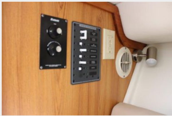
Cuddy Cabin 5 - AC Control
