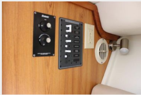
Cuddy Cabin 5 - AC Control
