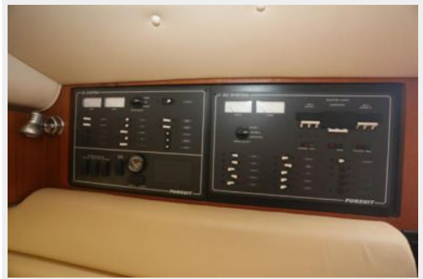
Main Distribution Panel
