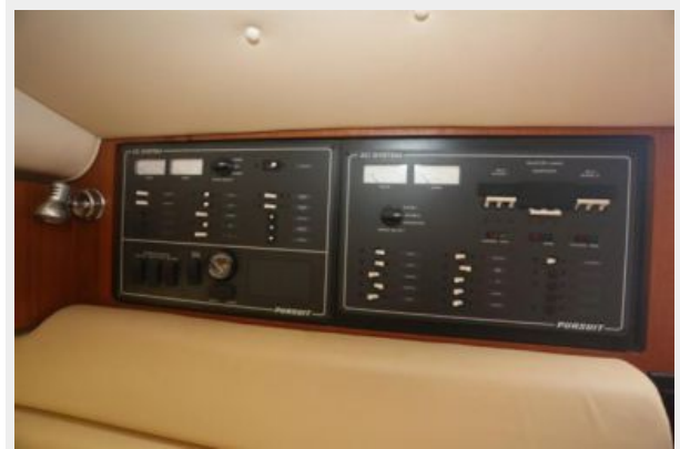
Main Distribution Panel
