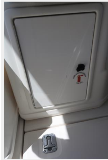
Fire Extinguisher Storage
