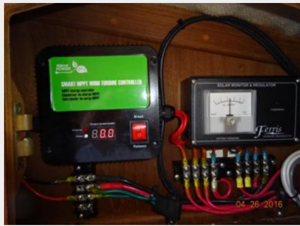
34' Pacific Seacraft electrical panels
