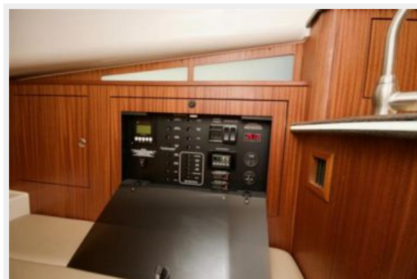
Main Distribution Panel
