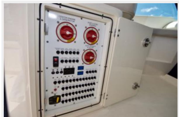
Engine / Generator Gauges
