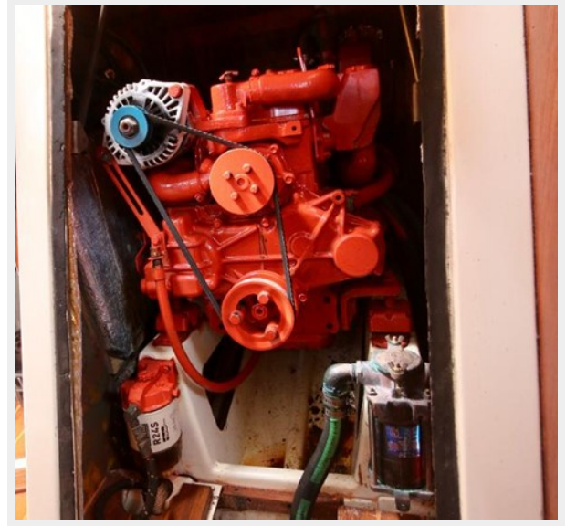
Engine access - 37 HP Westerbeke Diesel
