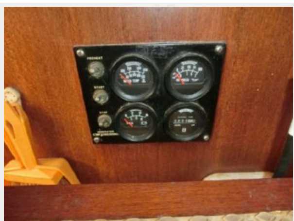
42' Whitby generator controls
