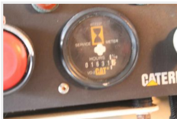
1631.7 Port Hr Meter 10/27/16
