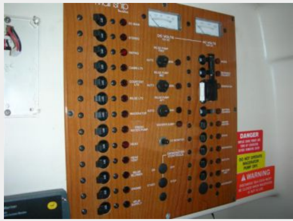
30' Mainship electrical panel
