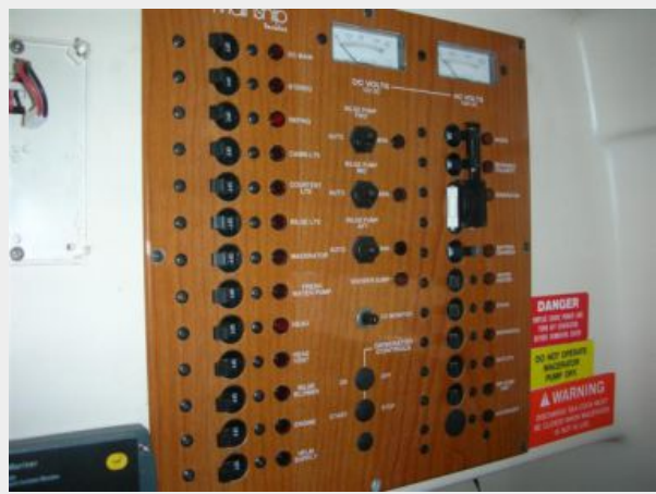
30' Mainship electrical panel
