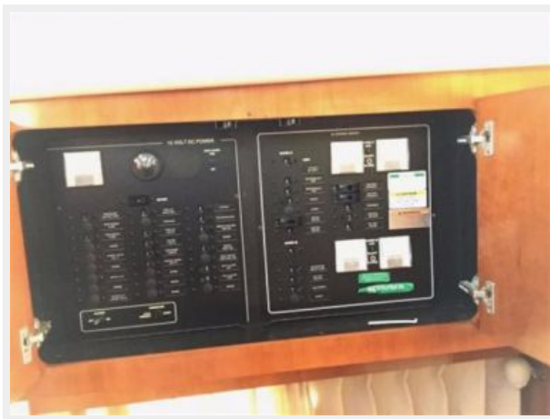
Circuit breakers on std side of salon.
