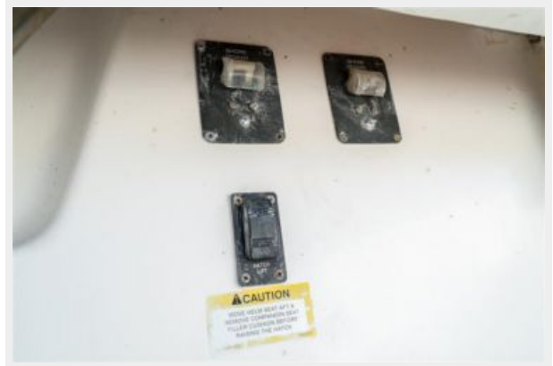
Hatch Lift / Shore Power
