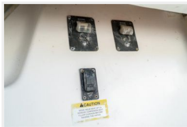
Hatch Lift / Shore Power
