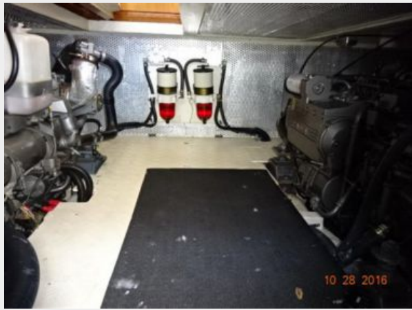
40' Albin engine room aft
