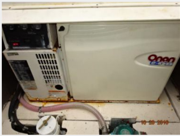
40' Albin generator soundbox
