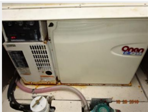
40' Albin generator soundbox
