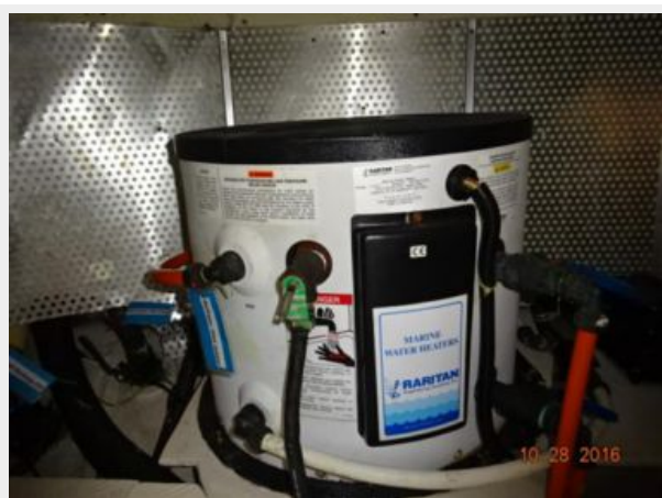
40' Albin water heater
