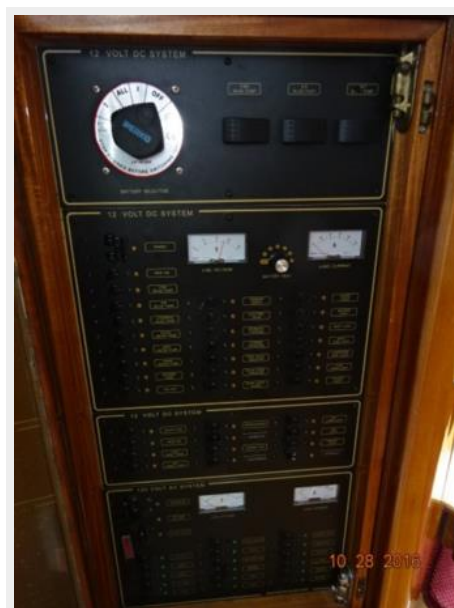
40' Albin electrical panel
