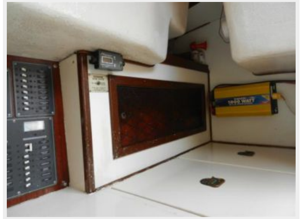
Electric panel, Cabinets, Invertor
