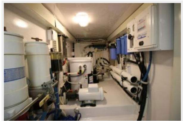
Forward Engine Room
