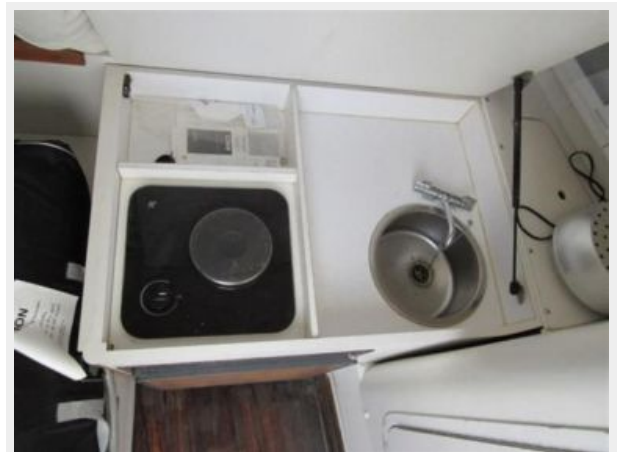
Accommodations 3 - Sink & Stove
