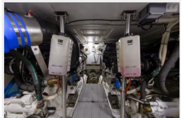
64' Azimut - Engine Room 1
