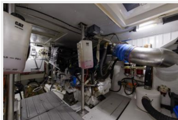
64' Azimut - Engine Room 3
