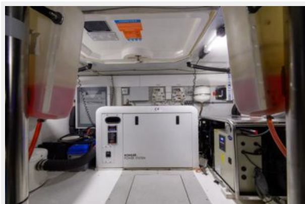
64' Azimut - Engine Room 4
