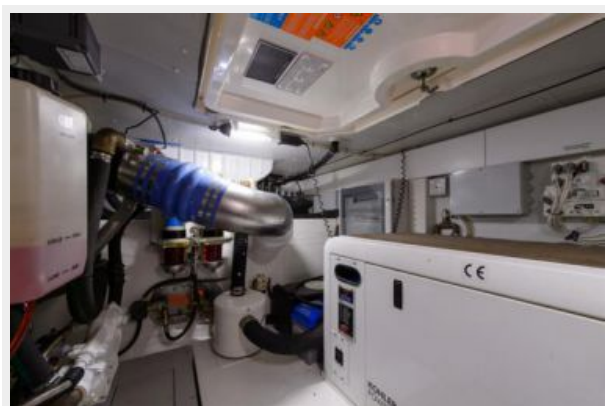
64' Azimut - Engine Room 6
