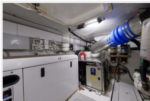
64' Azimut - Engine Room 5
