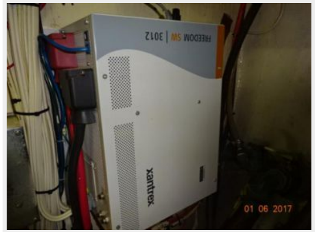
56' Nautical Developments inverter/charger
