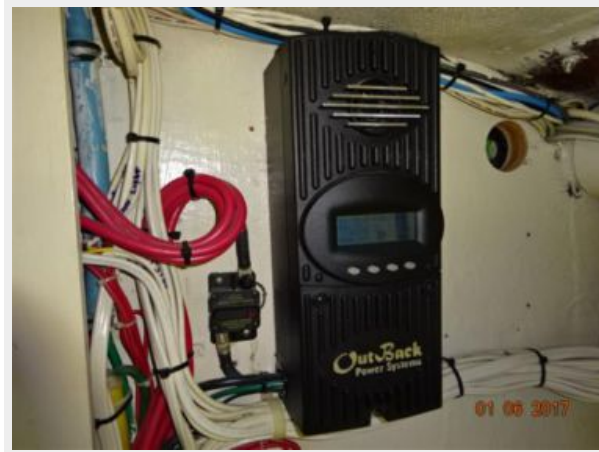
56' Nautical Developments solar panel controller
