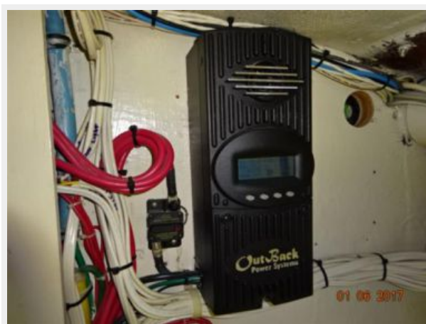
56' Nautical Developments solar panel controller
