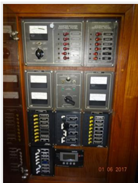
56' Nautical Developments electrical panels
