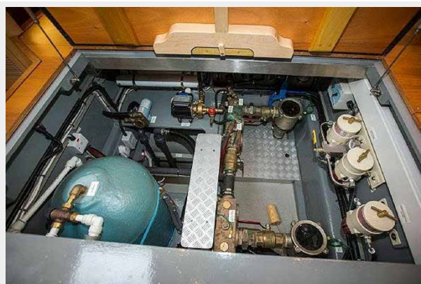
Easy Access to Plumbing
