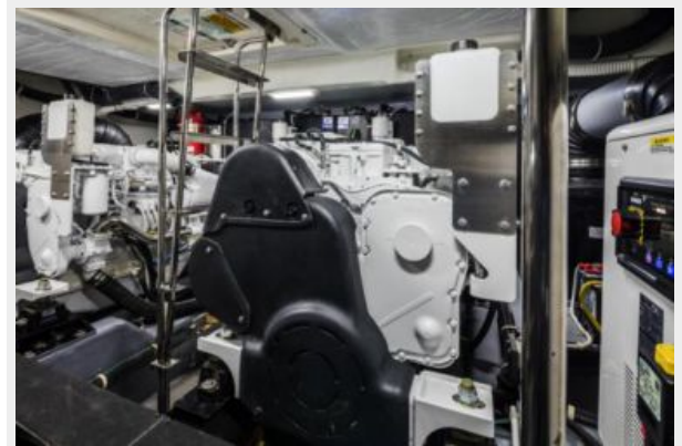
Carver C52 Engine Room
