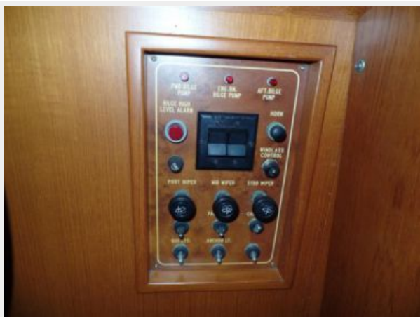
Lower helm controls.JPG
