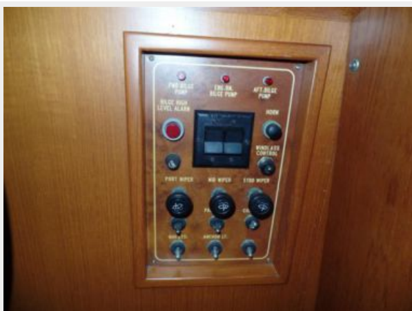
Lower helm controls.JPG
