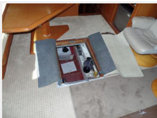
Engine room access.JPG
