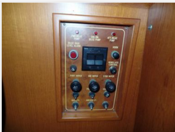
Lower helm controls.JPG
