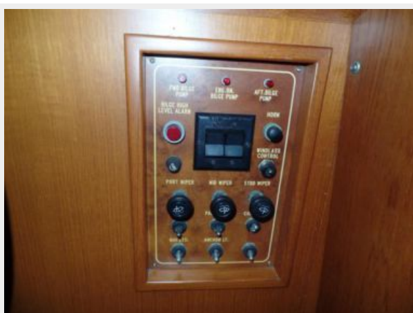
Lower helm controls.JPG
