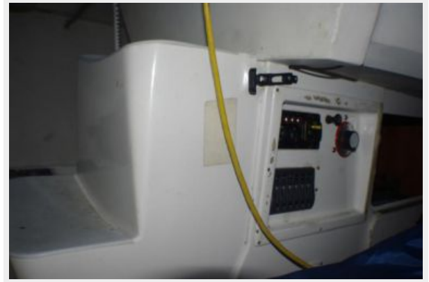
Battery switch and electrical panel
