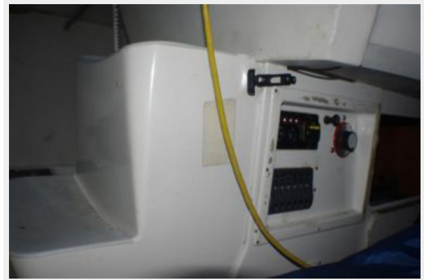
Battery switch and electrical panel
