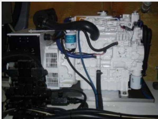
Phasor 12.5 kw Generator
