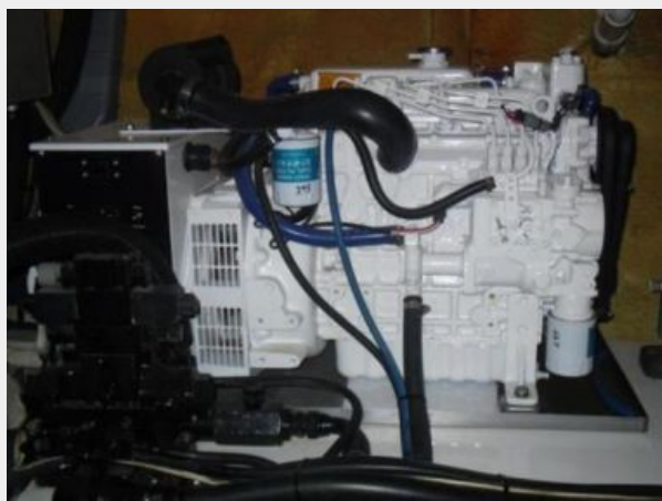
Phasor 12.5 kw Generator
