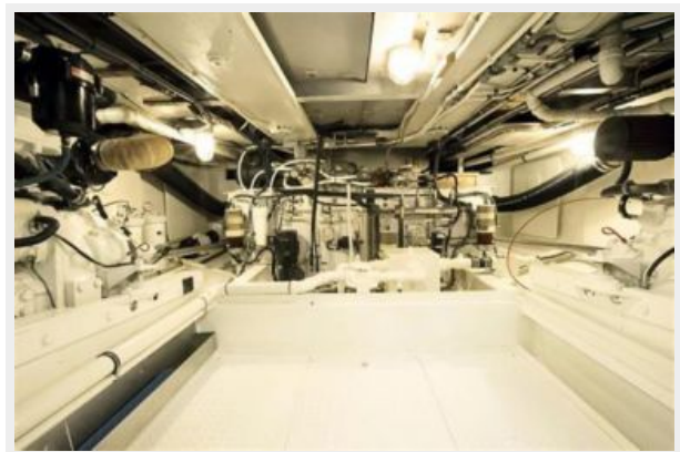
Engine Room Aft
