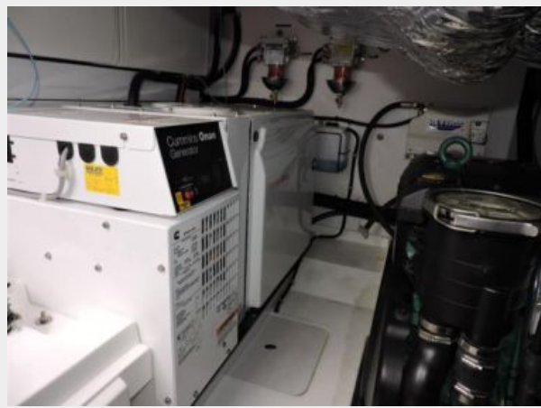
Engine Room Generator
