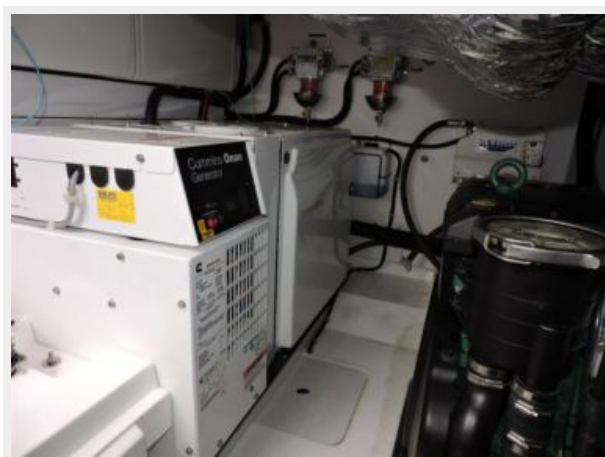
Engine Room Gnerator
